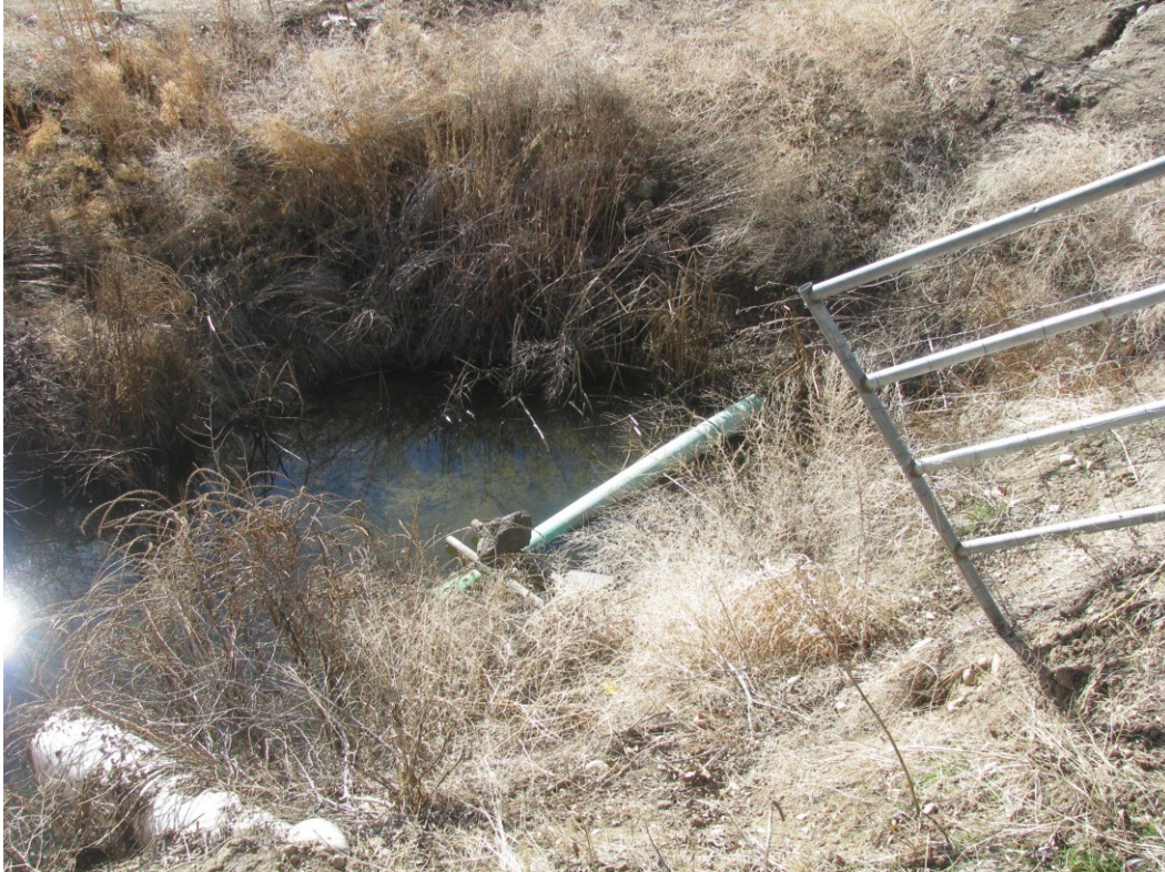
Figure 6. The historic drain ditch across the proposed Antelope Springs site has been filled in and an 8-inch PVC pipe was placed in an attempt to provide drainage for the Duesman site. The preliminary plat depicts this pipe as an existing condition, although the pipe was installed in 2012. (2/17/2013)
