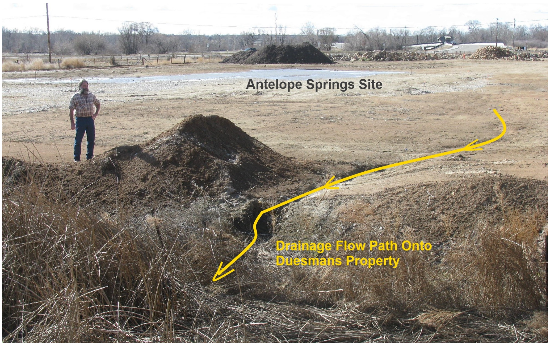
Figure 9. Since the Antelope Springs fill was placed, the adjoining pad has been graded toward the Duesman property and the new drainage ditch seen here was created. The new ditch is apparently intended to discharge drainage directly onto the Duesman property. As a direct result of the recently placed fill, the Antelope Springs property is approximately 3 to 4 feet higher in elevation than the adjoining Duesman property. Historic stormwater drainage from the Duesman site has been effectively blocked by this fill, which was extended into the original drain ditch in 2012. (2/17/2013)
