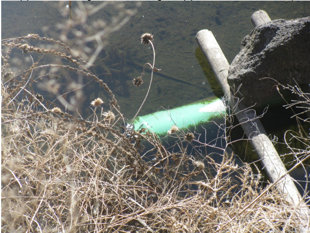
Figure 7. The 8-inch pipe is undersized for storm drainage purposes and lacks any trash rack. The end elevation is gravity controlled, utilizing a non-engineered and unique wood pole and large boulder contraption. Future storm drainage runoff from the Duesman property will be impacted by this recent alteration to the historic drainage system. (2/17/2013)
